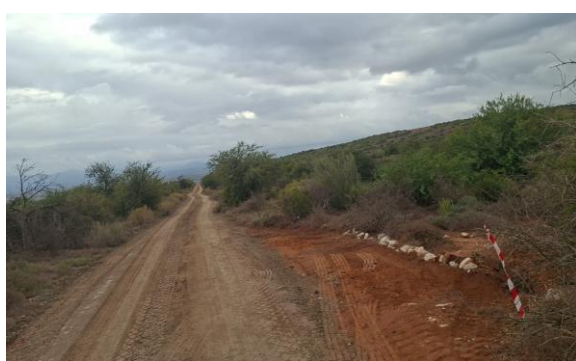
Figure 18: Example of temporary designated passing bay along narrow track to enable large construction vehicles to pass each other. Area must be clearly marked and rehabilitated once repair work is completed.
