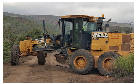
Figure 12: Example where grader drives off the road to make a u-turn or get out of the way of oncoming traffic.
