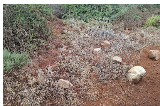
Figure 14: Example of area packed with large rocks and branches to support regrowth in an area where construction vehicles deviated from the designated turning and passing bays.
