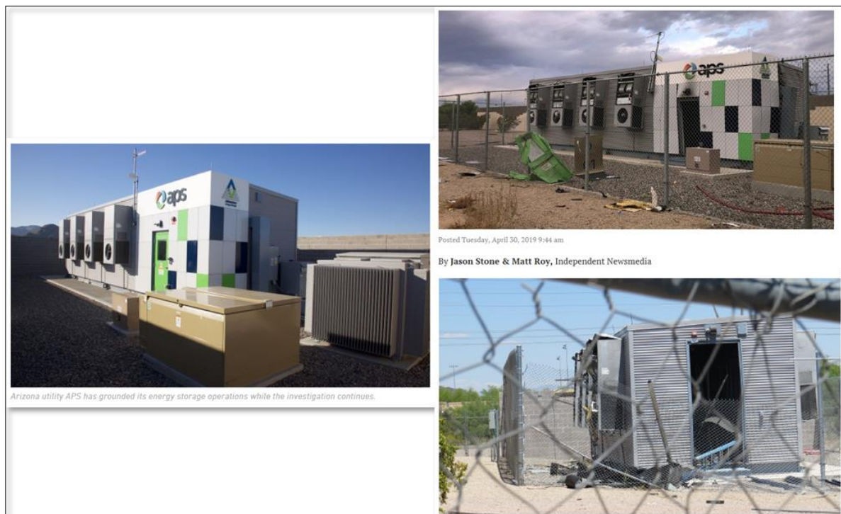
Figure 3.4.1 – Photo of lithium battery explosion scene
