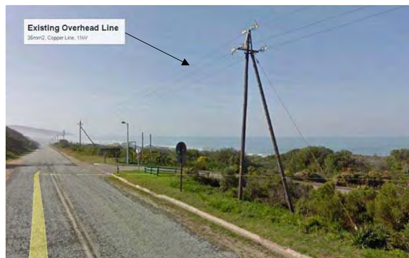
Figure 2: Existing 11kV Overhead Line
