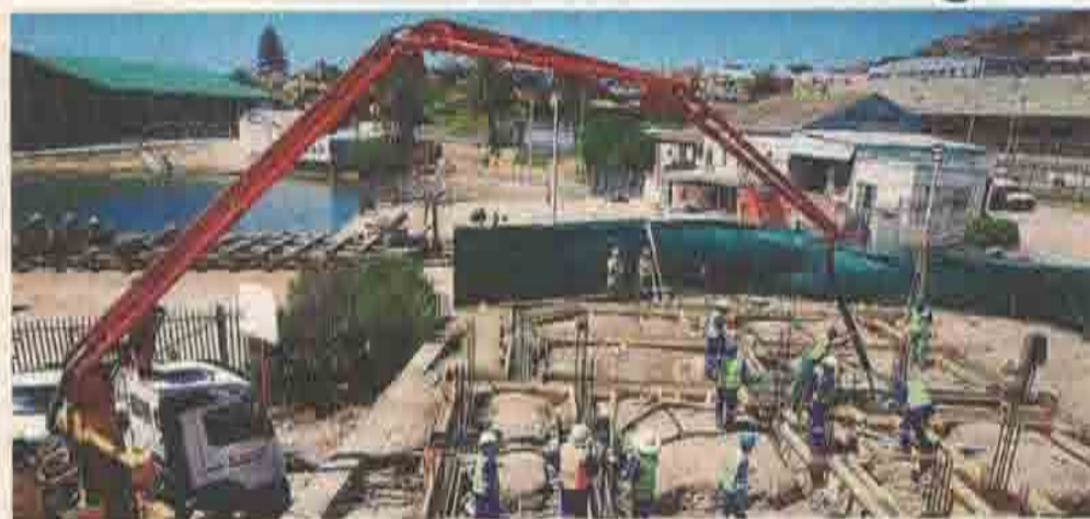
Port Manager, Shadrack Tshikalange, said the extension was essential as the port had continued to employ more people in line with Transnet's Market Demand Strategy (MDS), which aimed to create jobs and drive economic growth.
