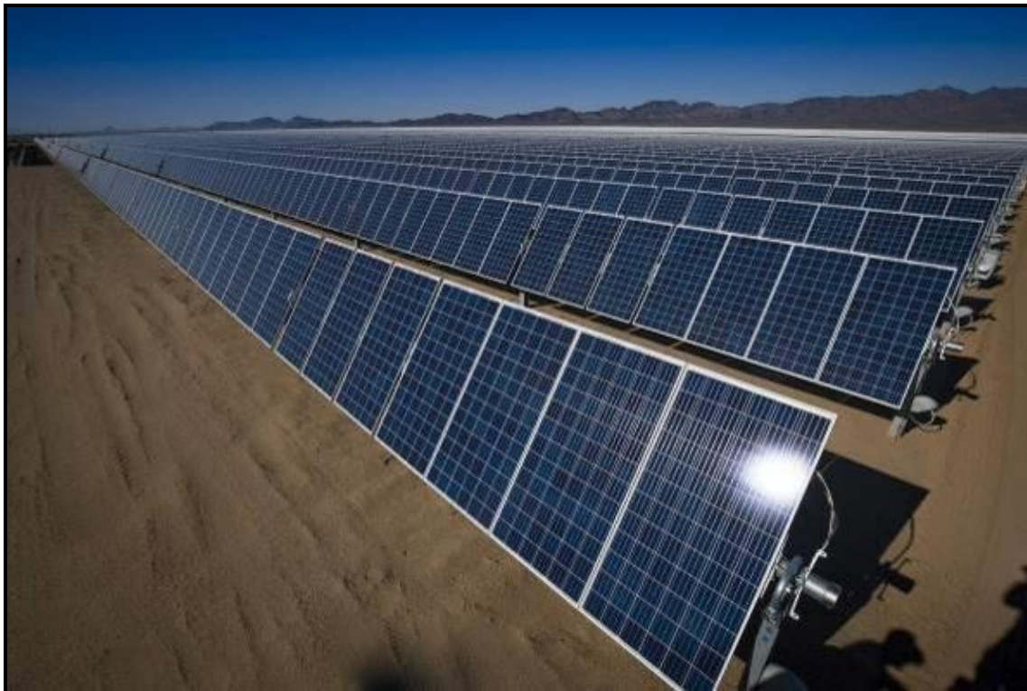
Figure 1.2: Typical PV SEF facility
