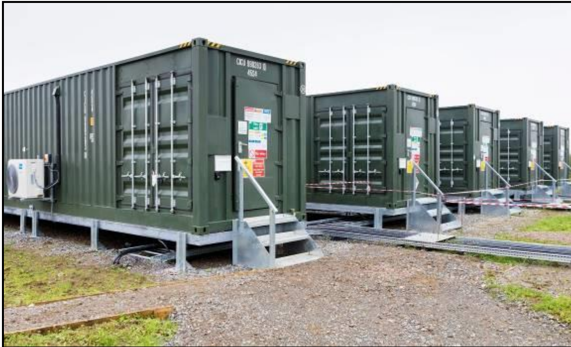
Figure 1.3: Example of BESS located in storage containers
