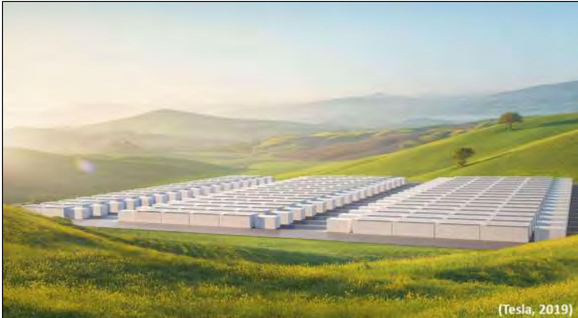
Figure 1: Tesla's Megapack Li-ion Battery (Modular System).
