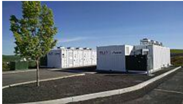
1 MW 4 MWh containerized vanadium flow battery owned by Avista Utilities and manufactured by UniEnergy Technologies
