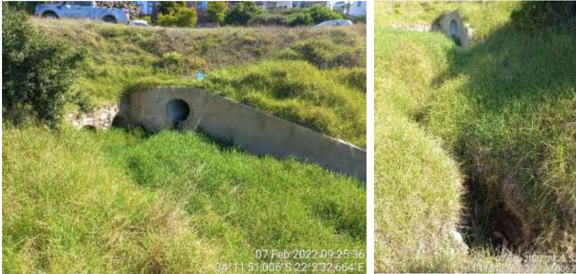
Figure 5: Ferox Street culvert & erosion gully below it.
