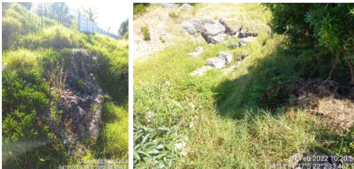
Figure 4: Failing bank stabilisation structure - view up & down eastern bank.
