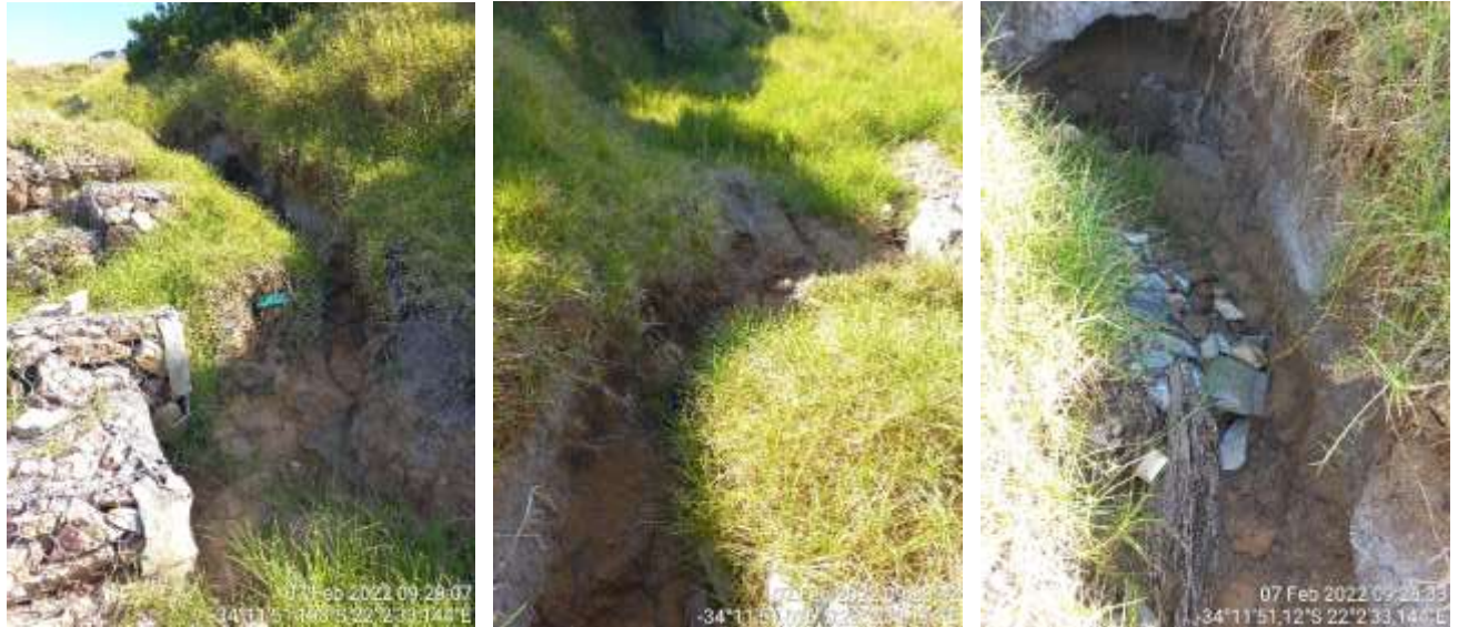
Figure 3: Failed gabion structure & bypass erosion gully undercutting eastern bank.
