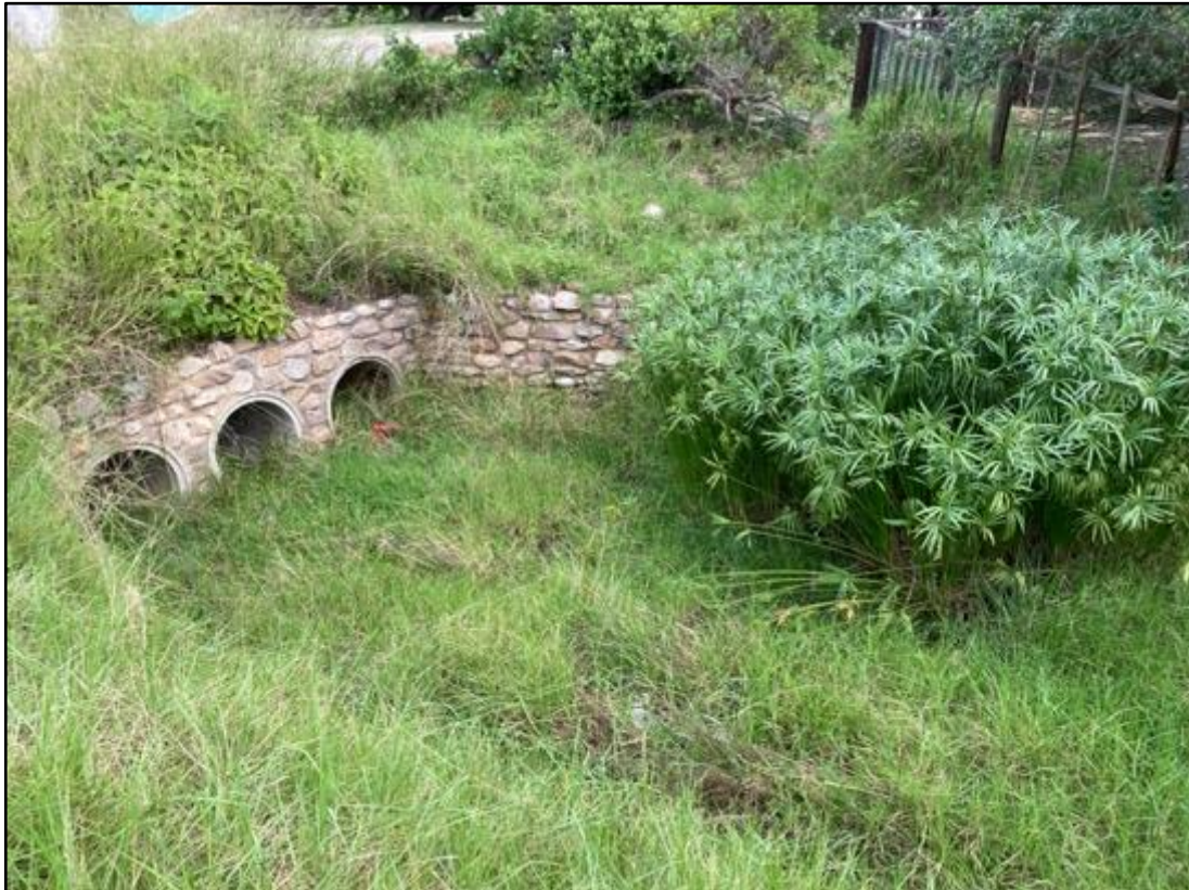
Figure 8: Culverts at the bottom end of the site showing kikuya grass dominating.
