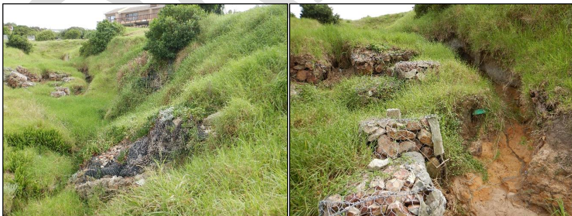
Figure 6: Photographs illustrating failed gabion structures and erosion of the eastern embankment.
