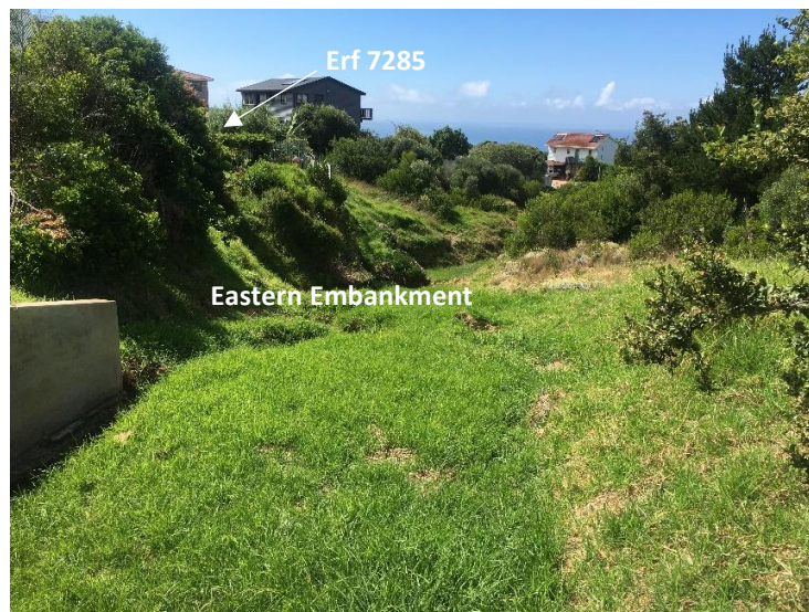
Figure 4: Eastern bank of watercourse undercut by erosion.
