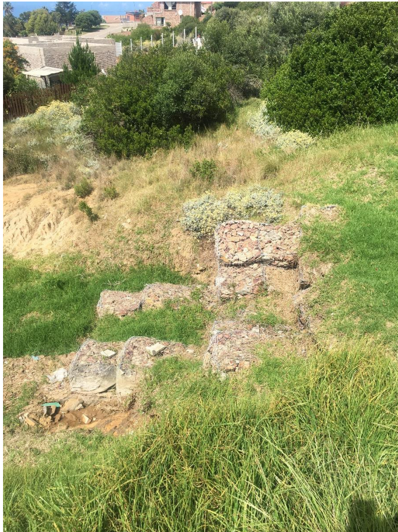
Figure 2: Failed upstream gabion weir structure.
