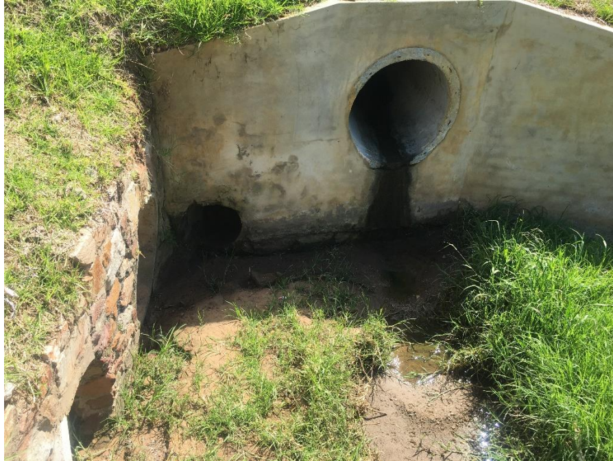
Figure 6: Lack of maintenance resulting in silt build-up and vegetation overgrowth.
