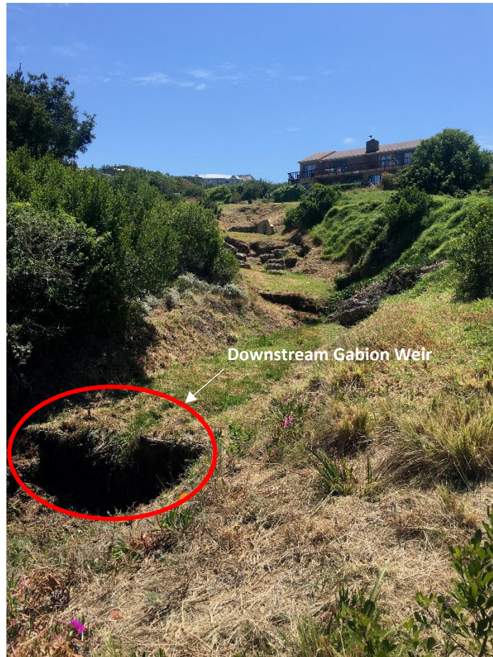
Figure 3: Partially failed downstream gabion weir structure.
