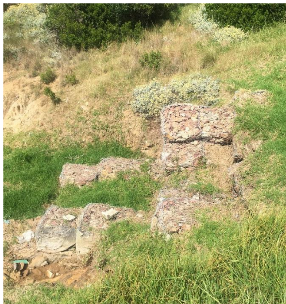
Figure 4: Failed displaced weir structure, A. Ferox.
