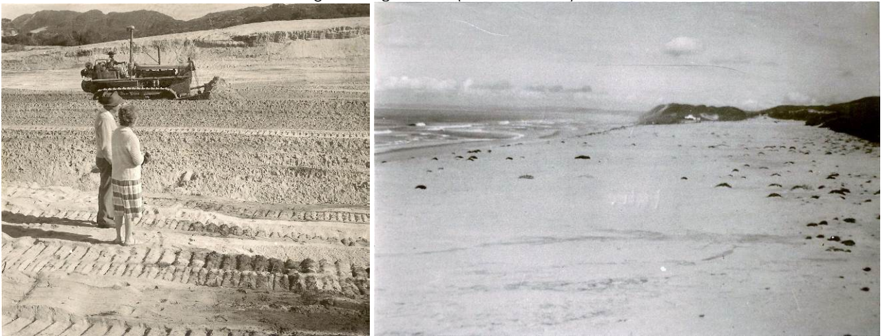
Image 1 (left): Coastal dunes being bulldozed (1959) in preparation for construction of Dwarswegstrand resort (Truster Family) Image 2 (right): Same transformed area (1964) prior to commencement of construction of Dwarswegstrand resort (Olivier, F).
