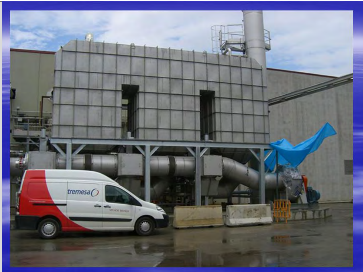
Figure 45: Regenerative Thermal Oxidiser (Tremesa, 2019)
