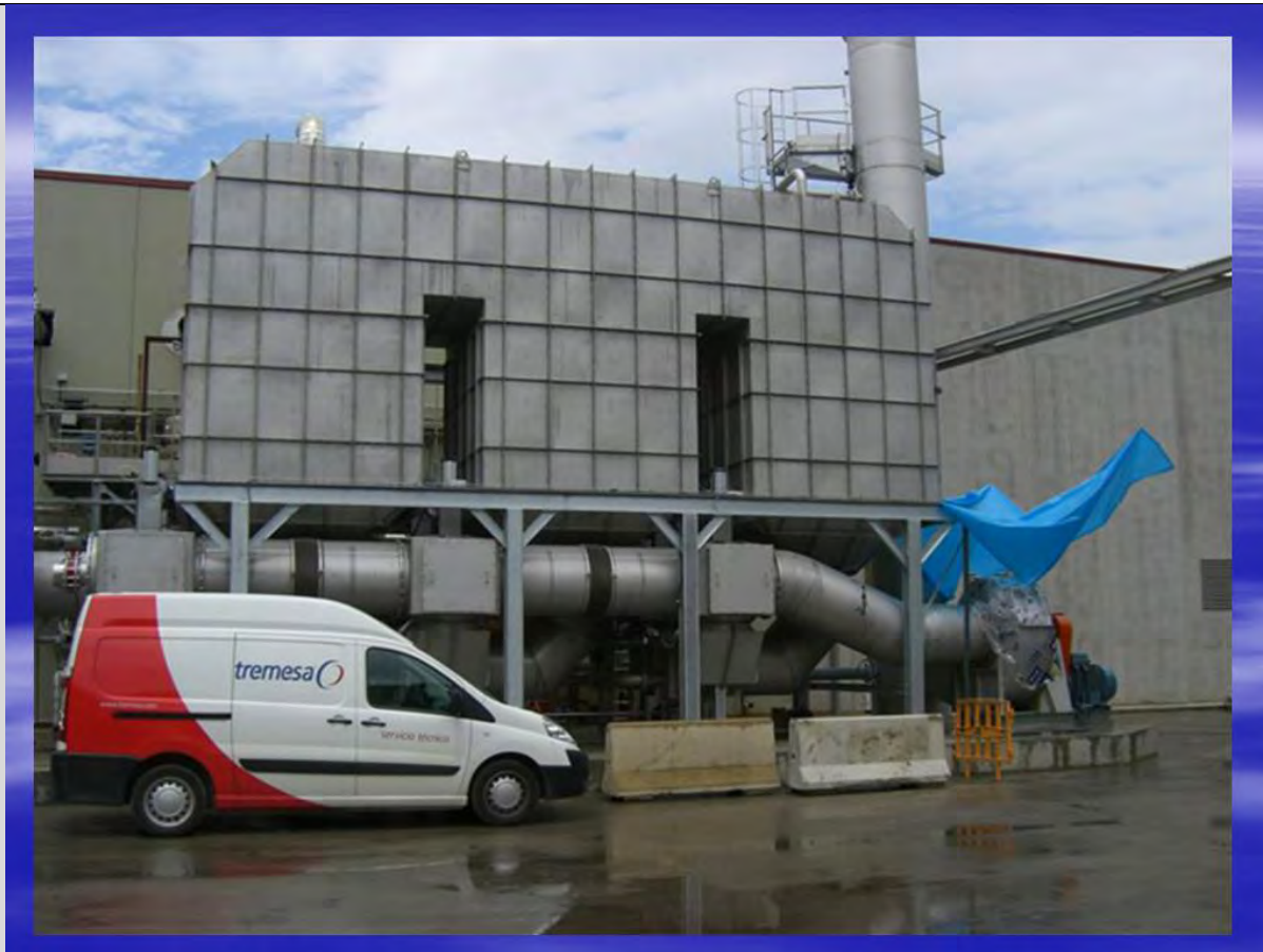
Figure 22: Regenerative Thermal Oxidiser (Tremesa, 2019)
