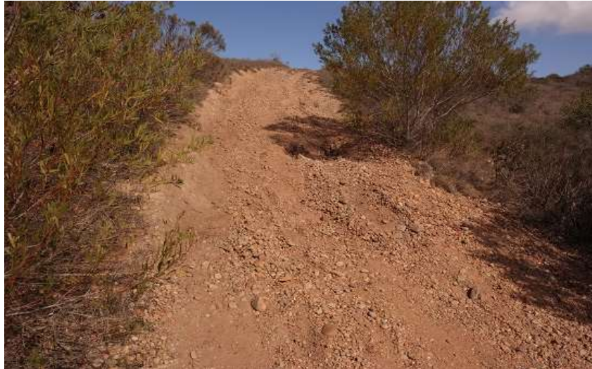
Plate 8: Steep and eroded access to the area, caused by offroad vehicles, going west, off Kameeldoring Avenue.
