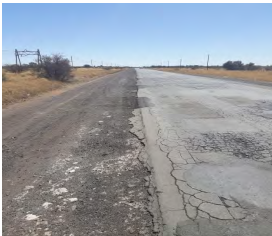
Photograph 3.5: non-existing road edge
