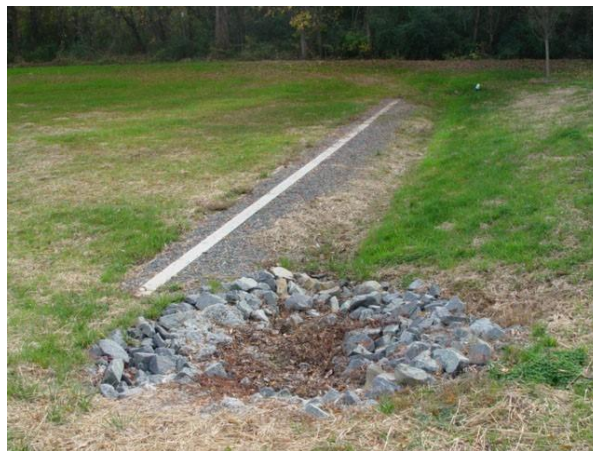
Figure 17. Example of a level spreader with the outflow section protected by rip rap.
