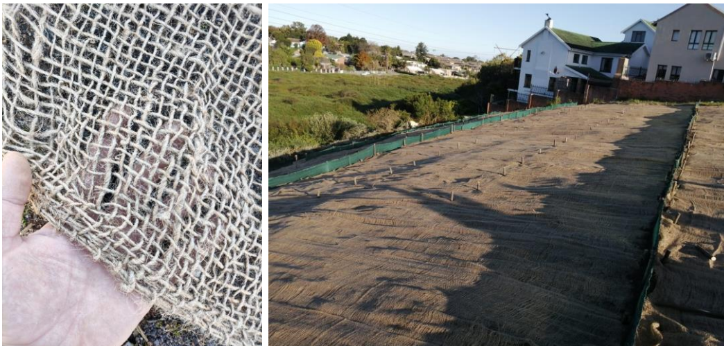
Figure 16. Example of jute mesh also known as soil saver matting placed on a slope seeded with oats and further protected with silt fencing.
