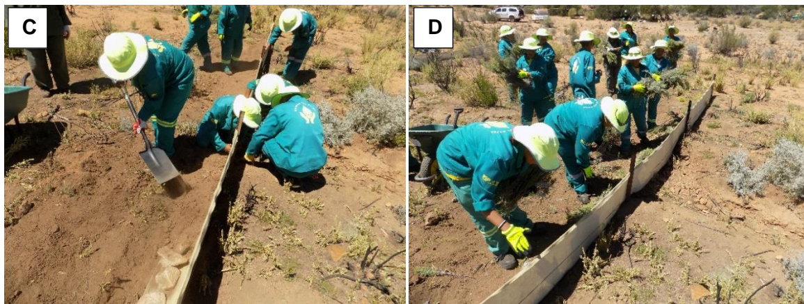
Figure 18. Installation of the soil erosion control fence. A: Installing the standards and wires and preparing the trench. B: Fitting the geotextile, tying it on with wire. C: Filling in the trench over the geotextile. D: Applying a mulch against the completed fence (Photos courtesy Ken Coetzee).
