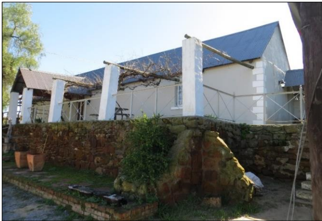
Figure 34: South-eastern corner of the older house on its large stone plinth (waypoint 440).
