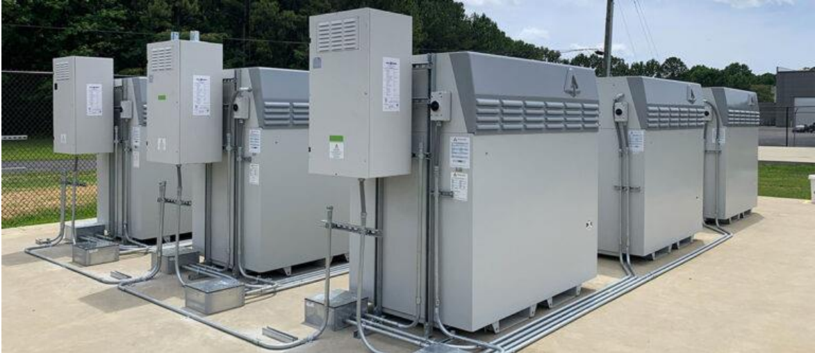
Figure 4. Example of a Photomontage Vanadium Flow Batteries in landscape (US Vanadium, n.d.)
